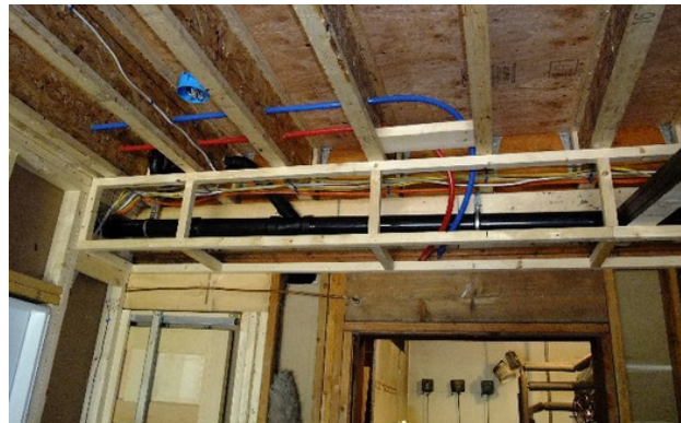
Around raceways and chases that are usually closed with a bump-out
